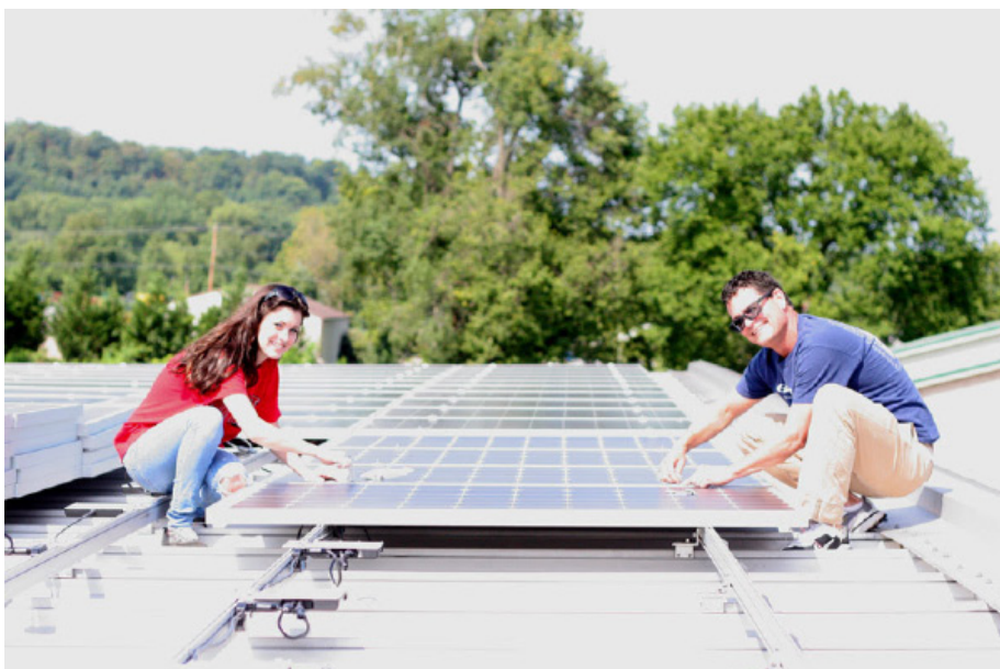
In Williamson, there are panels installed by laid-off coal miners
